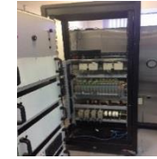
Topside PLC, Surface Modem & Subsea Gateway Test Setup
